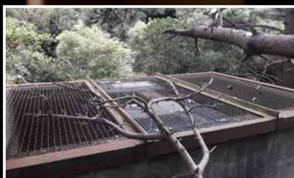
The top of the vertical vent above the tunnel. Note the dead growth around the tunnel vent.
