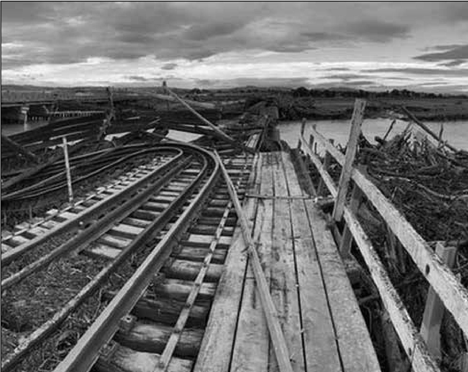
Cyclone Gabrielle caused significant damage to Rail infrastructure. Bridge 217 (pictured above) on the Palmerston North/Gisborne Line was washed away.
